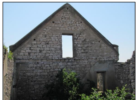
Figure 26: Inside view of the still standing north gable showing the concrete lintel above the loft door.
