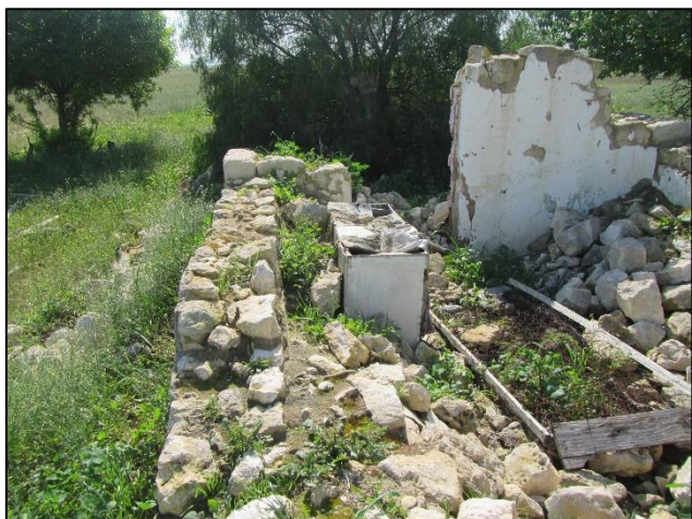
Figure 18: The ruin at waypoint 235 the walls made with two calcrete skins and a rubble fill.
